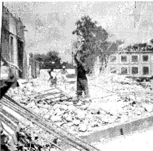
Construction worker destroying the mill building, Marienthal, Austria, ca. 1931, unknown photographer [possibly Hans Zeisel], Marie Jahoda Papers 41/F104, AGSÖ Graz
