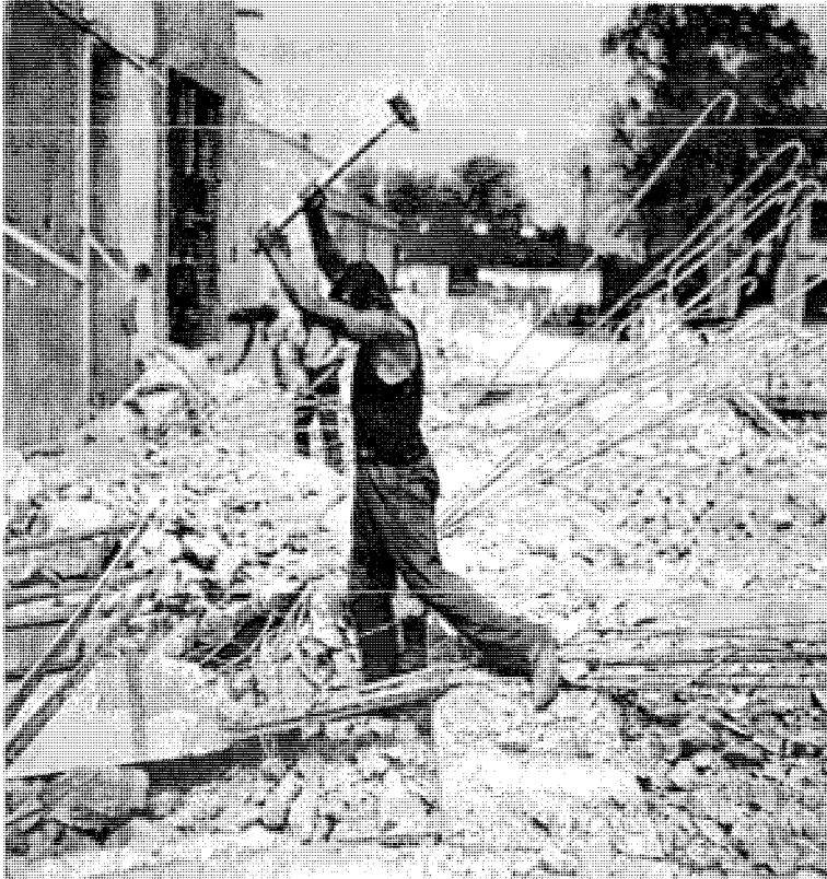
Construction Worker destroying the mill building, Marienthal, Austria, ca. 1931, unknown photographer [possibly Hans Zeisel], Marie Jahoda Papers 41/F-103, AGSÖ Graz
